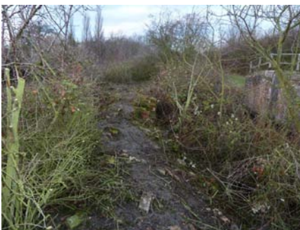
The trees and brambles on the right, growing out of what was the offside wall of lock 14
